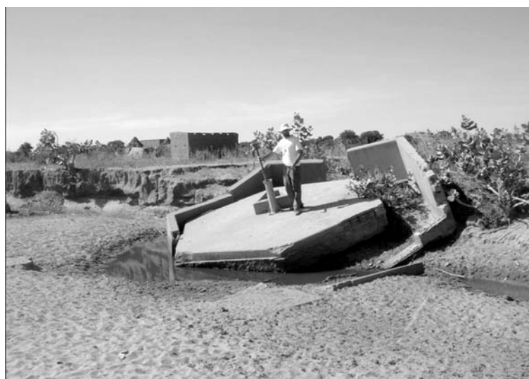
Figure 5: Total collapse of well infrastructure due to seasonal flood erosion, near the village of Abdi in eastern Chad. This can be prevented by locating production wells outside of a wadi, along fractures fed by the wadi's deep reservoir.
